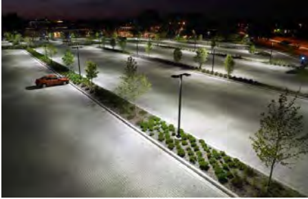
Parking lighting with LED luminaries at Johnson Controls campus, Glendale, WI
